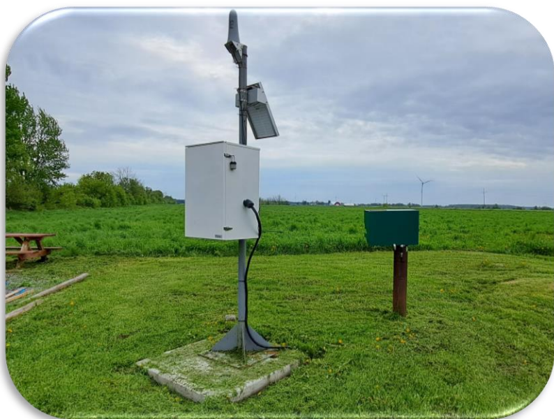
Berwick station with new FTS box installed North Stormont
