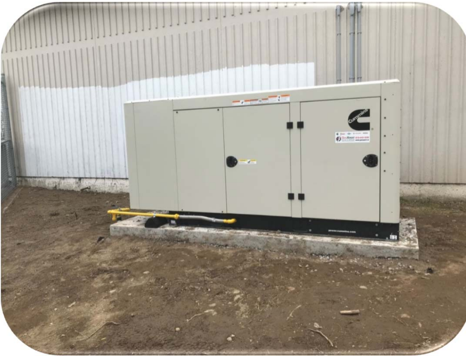
New generator, Chesterville Dam North Dundas
