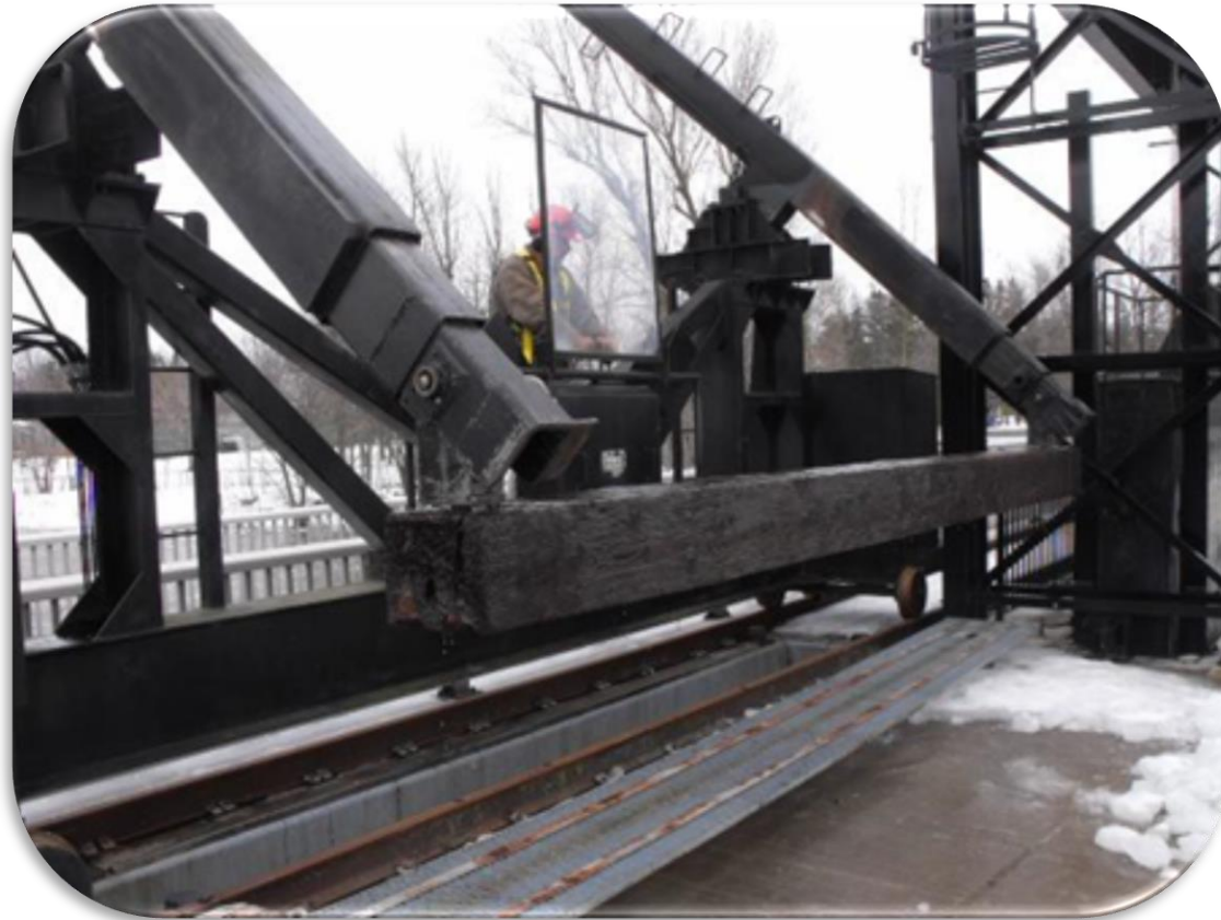
Log Lifter removing stop log at Chesterville Dam
