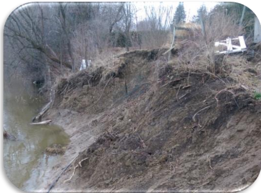
Erosion on private property, Embrun, Ontario, 2017
